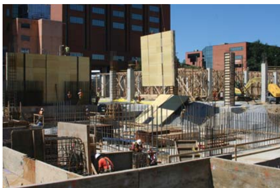
Construction workers use a tower crane to carefully lower a wall into place on the site of the new Le Bonheur Children's.
