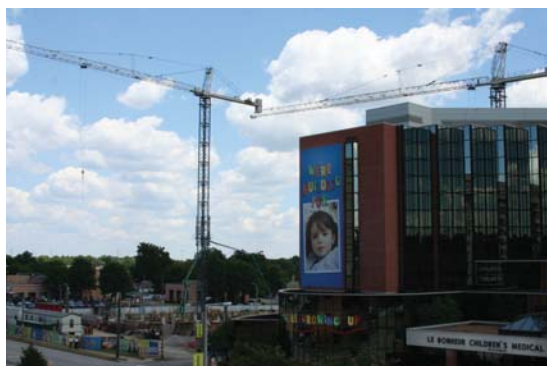
Two 14-story tower cranes frame the existing Le Bonheur Children's and the site where the new hospital is under construction.
