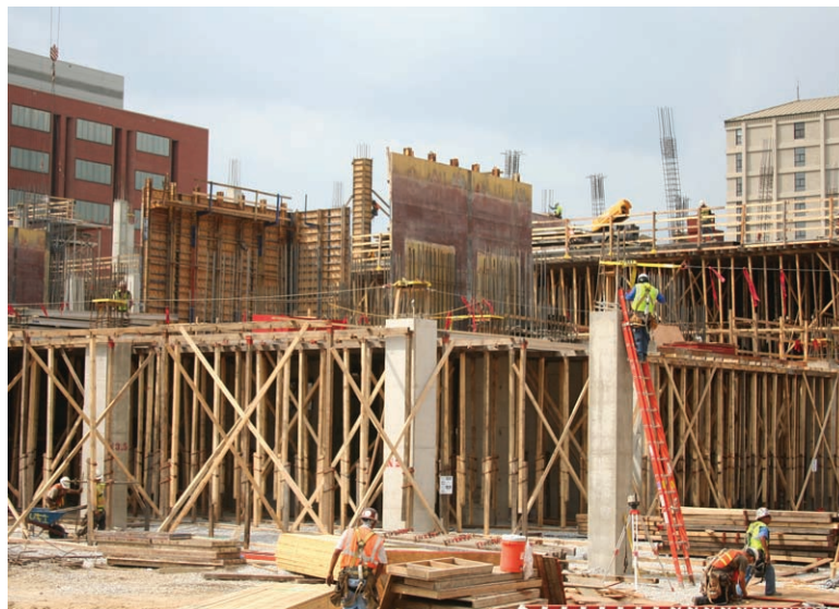
Workers at the new Le Bonheur construction site have begun building the frameworks for concrete pillars to support the first several floors of the hospital. The hospital has been designed with input from families.
