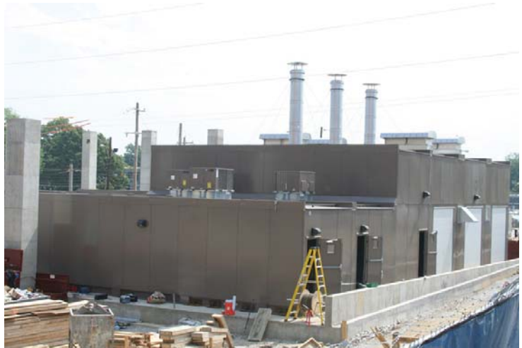
The central energy plant on site at the new Le Bonheur will supply the hospital with power in a highly cost effective and energy efficient way.
